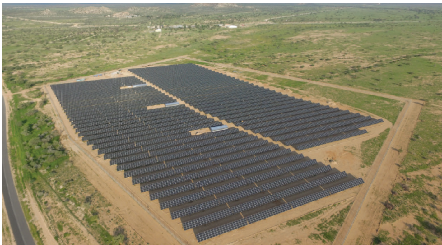
Figure 10: Project S-PV 6 (5MW Solar PV power plant, Karibib, Namibia 14 )
